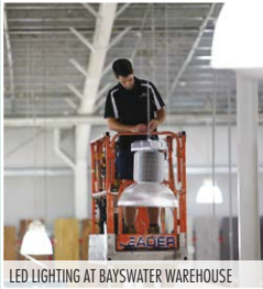
LED LIGHTING AT BAYSWATER WAREHOUSE
