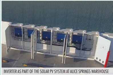
INVERTER AS PART OF THE SOLAR PV SYSTEM AT ALICE SPRINGS WAREHOUSE
